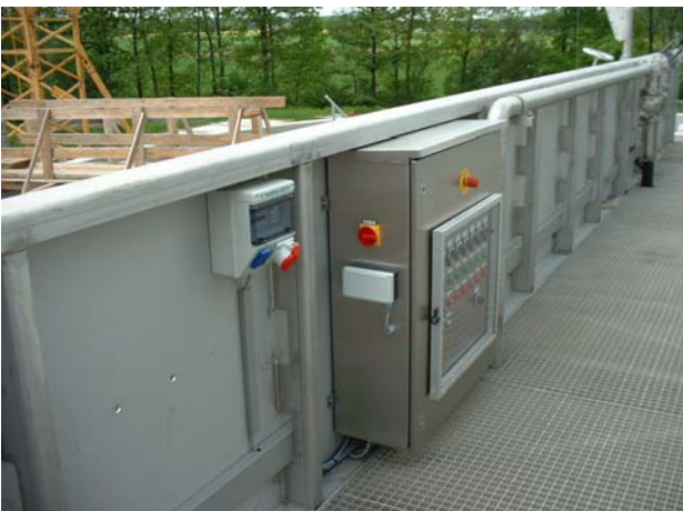
Control panel made of stainless
