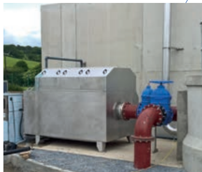
MSS B10-1500 – tank version outdoor installation
