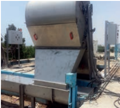
Step chain screen with screw compactor
