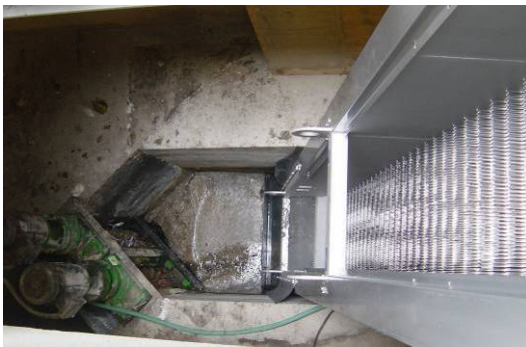
Figure 8- Deep Channel SSV at Rhinelander, WI (Replacing a grinder)
