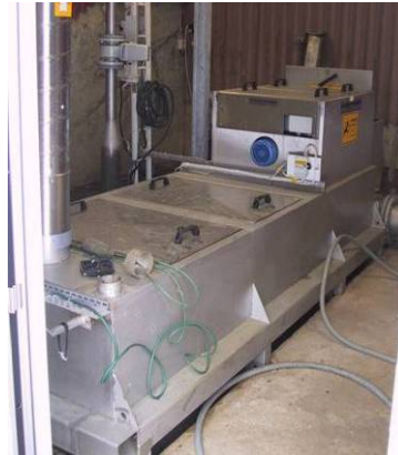
Figure 15 – Tank mounted Step screens
