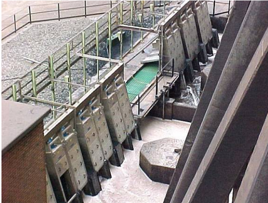
Figure 14 – SSV for cooling water intake
