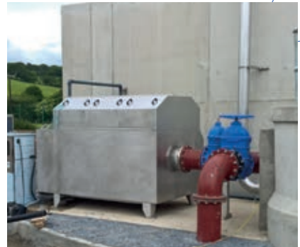
MSS B10-1500 – tank version outdoor installation
