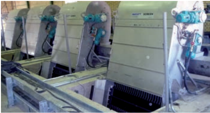
2000-BS-2000 with screw conveyor, 4 out of totally 12 installed
